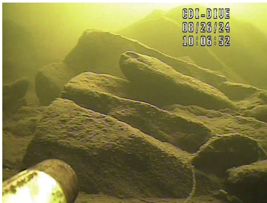
Photo 5-4 Boulders and Debris Observed Underwater at the Upstream Face of Bar Mills Dam
