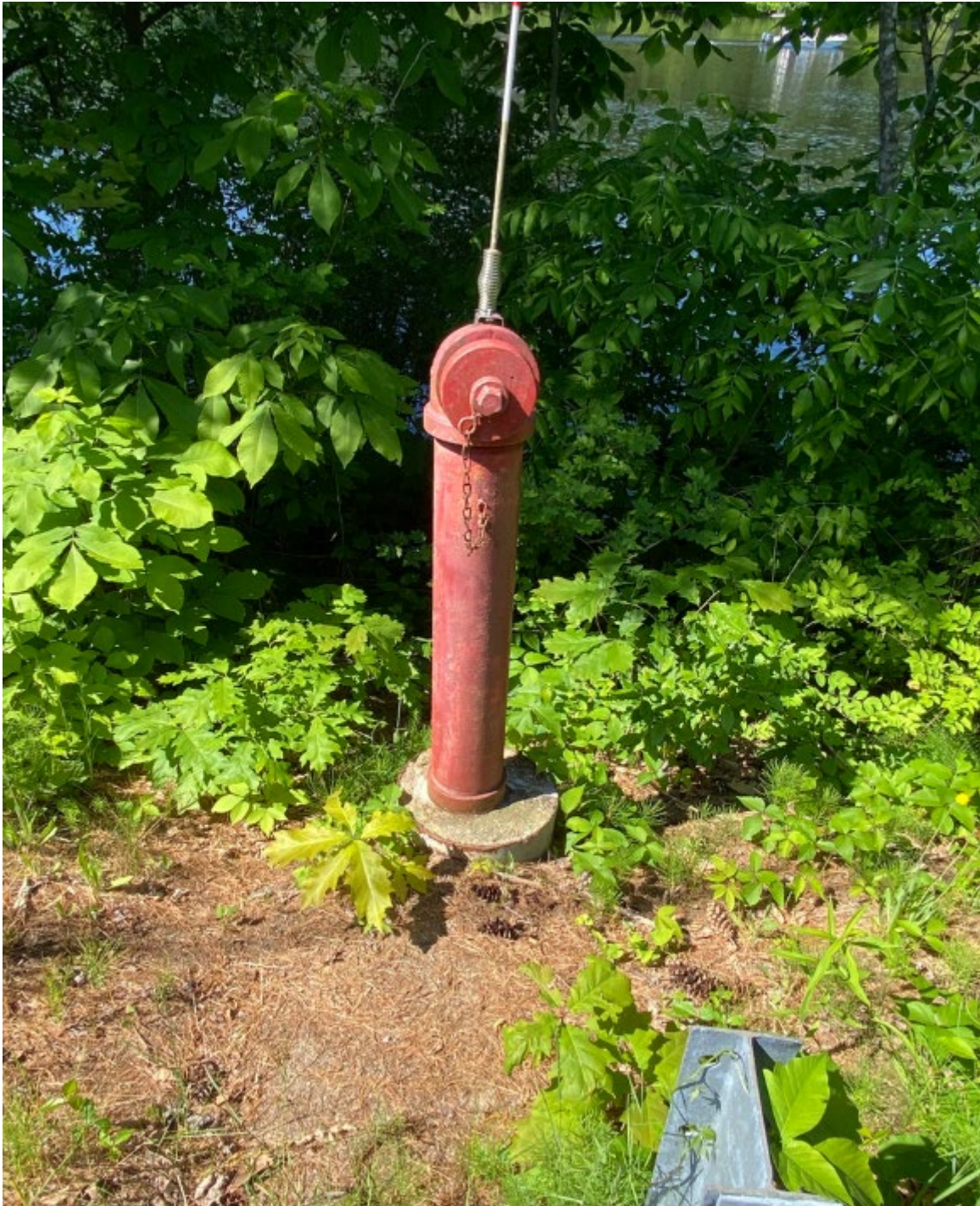
Photo 2-4 Existing Dry Hydrant on Depot Street in Buxton
